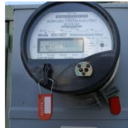
kWh meter with seal
